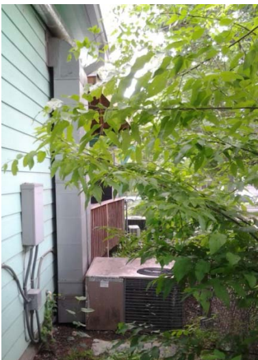
Figure 3.7- Exterior HVAC fan units with exposed ductwork.
