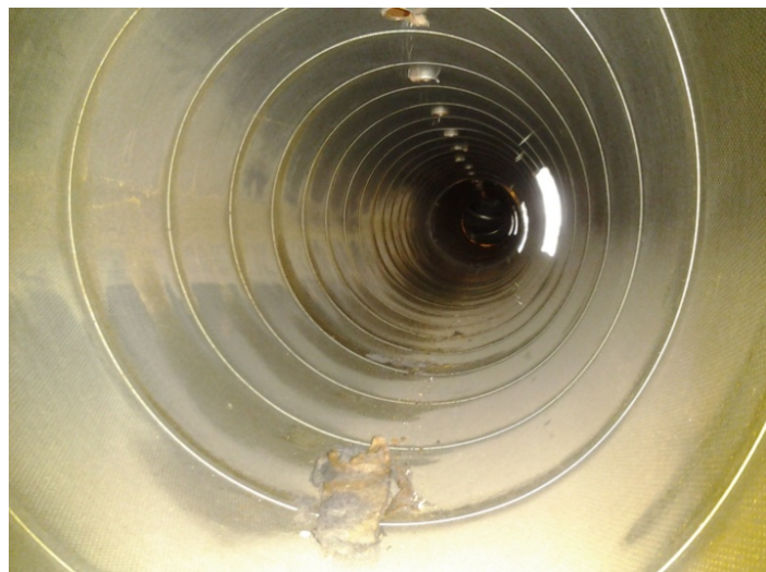
Figure 3.8- Inside of Tracking Room ductwork, note lack of internal lining.
