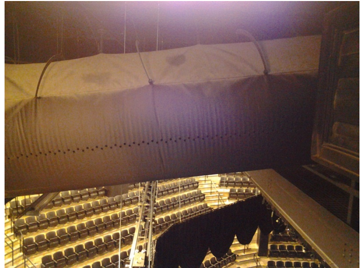
Figure 5.7- Fabric ductwork serving main seating area
