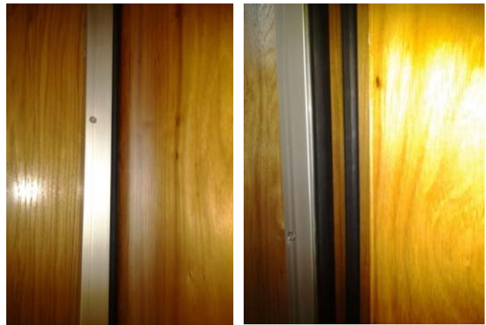
Figure 4.7- Adjustable door seals at Vestibule/ Tracking Room door – door closed (left) and door open (right)
