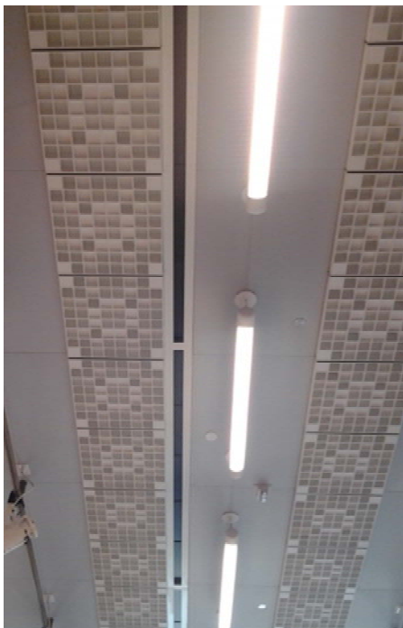
Figure 4.3- Ceiling mounted acoustical diffusers
