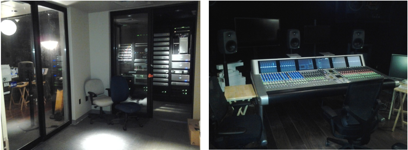
Figure 5.2- Interior views of the Audio Control Suite – Vestibule, with Control & Machine Rooms visible (left), console and near-field monitors (right)
