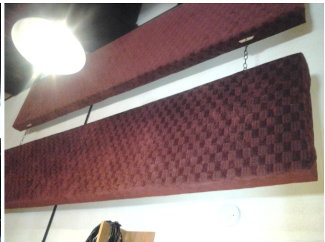
Figure 2.4- Acoustical absorption at the wall is hung from the ceiling with an airspace behind
