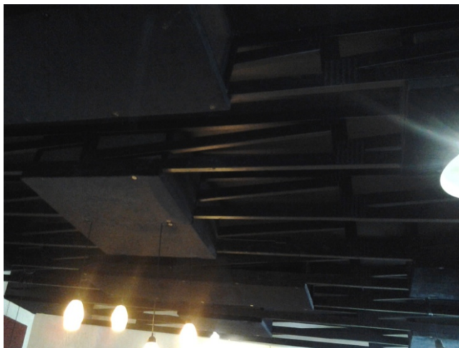
Figure 2.3- Acoustical absorption installed at the ceiling
