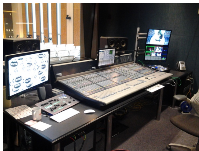
Figure 4.1-Interior of the Tracking Room from the northeast (top) and southwest (middle) corners, and the Control Room (bottom)
